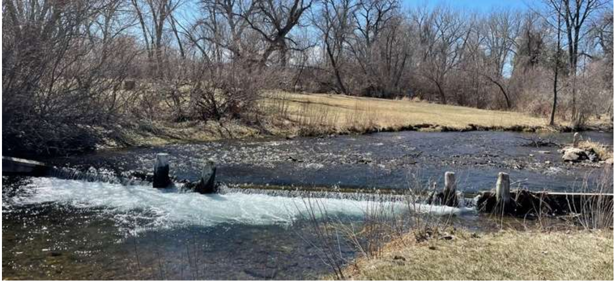
Figure 15: Smaller diversion structures that can be a hindrance to navigation and a life-safety issue are in the reach.
