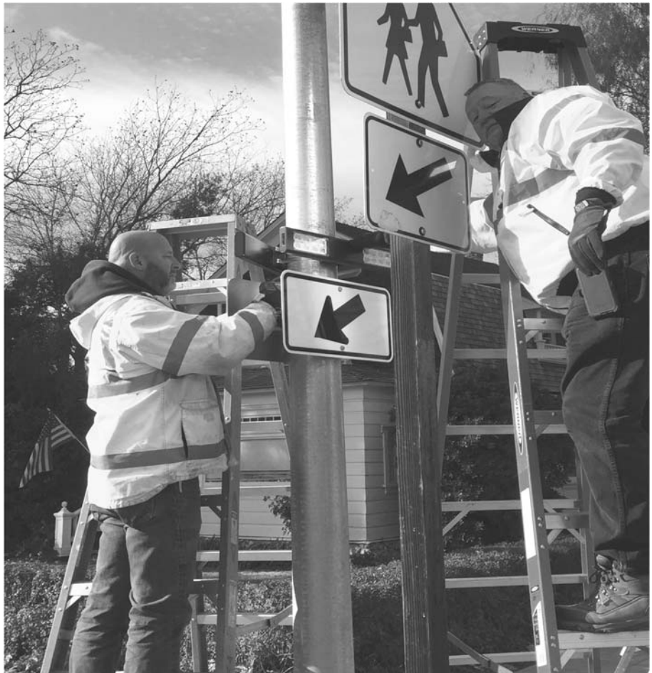
Pictured above are Steve Johnson and Joe Tremaine of West Coast Electric from Santa Rosa, CA installing the Solar Crosswalks in Esparto.
