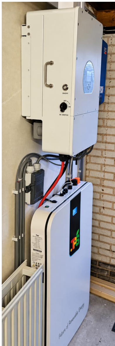
HomeSystem: 12kW/ 14kWh
