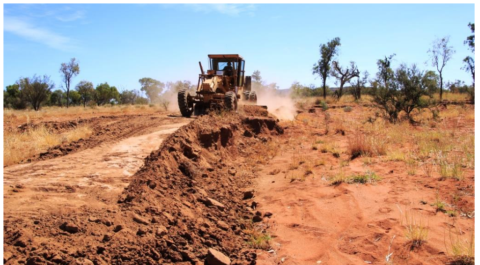
Sides of gully which flowed from the head of the erosion. Removing the sharp edges and battering them flat
