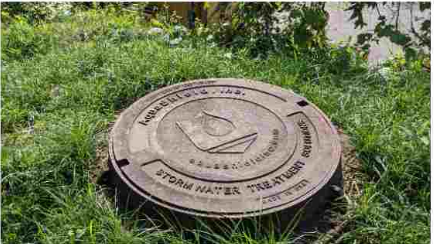
Aqua- Swirl immediately west of the North Outfall at Portage Creek.
