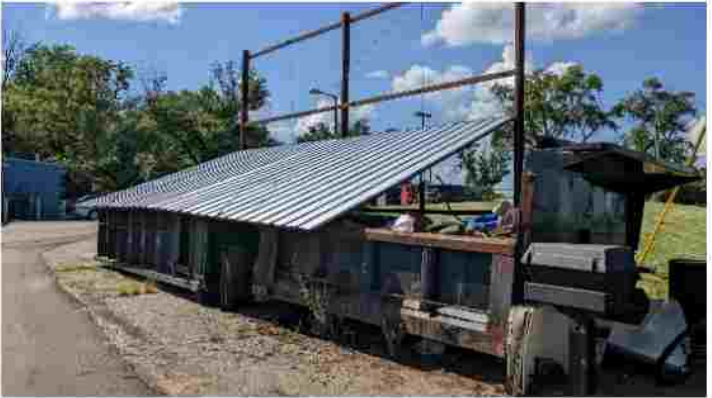
Metal Recycling Bin South of Fueling Station (see Figure 2). Area is covered to prevent seepage from rainwater.
