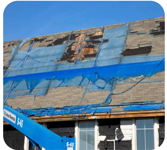
Structural damage to the roof of the Camp Johnson Chapel on Camp Johnson, North Carolina, Nov. 21, 2019. The chapel, built in 1941, is undergoing historical preservation and reconstruction projects after sustaining significant damage caused by Hurricane Florence in September 2018. • Photo: Lance Cpl. Ginnie Lee, U.S Marine Corps
