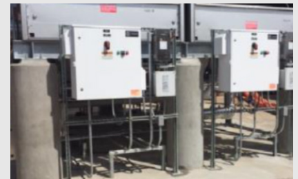
Mechanical and Fire Suppression Altus AFB, OK, USACE Tulsa
