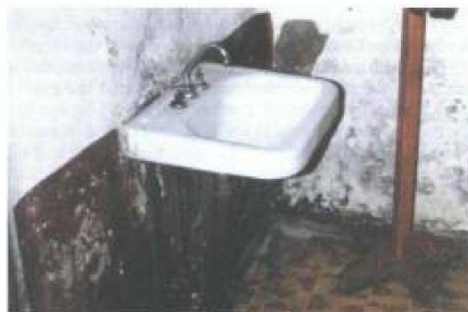
Washing facilities in a children's hospital ward
