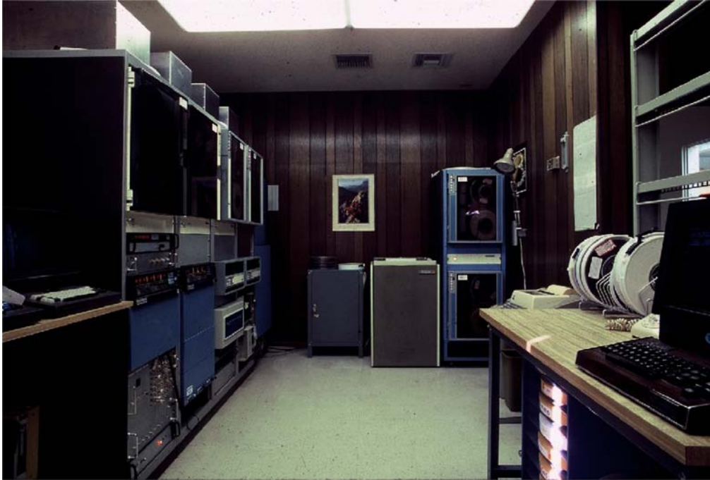
Figure 21. Computer room, processors, tape drives, and disk drives.
