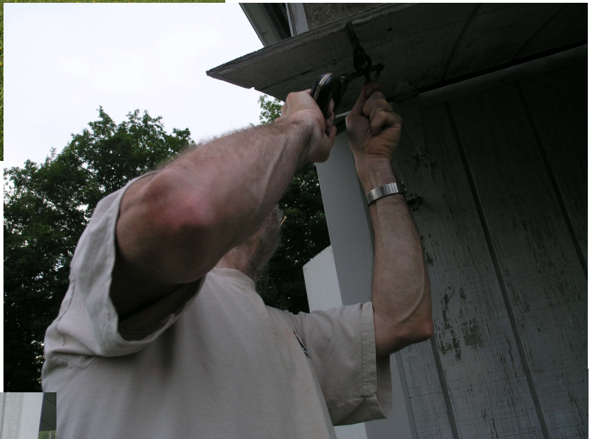
Right: Dan Rothstein working to replace the pull bar on the south wall flap.
