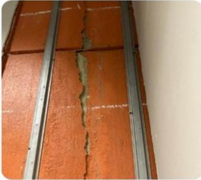
Cracks in Foundation
