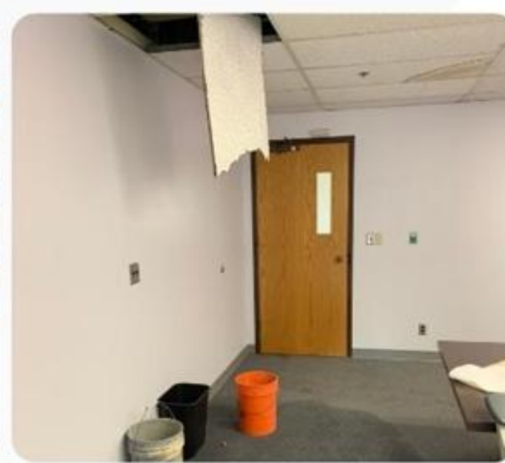
HVAC Pipe Failures
