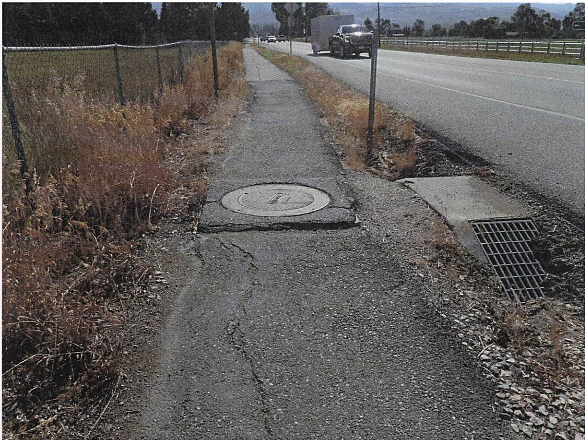
Figure 20: Uneven pavement in side path near Mountain Green
