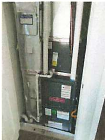
Upper Level Furnace
